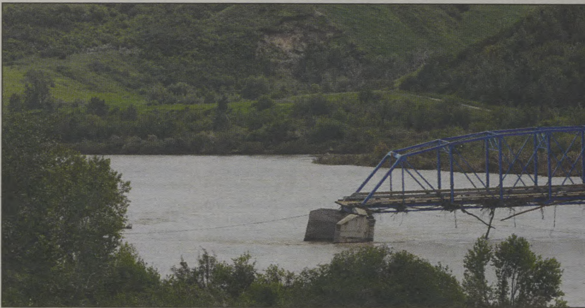
The Chicago Bridge across the Bow River at Siksika was badly damaged preventing travel between parts of the community.
